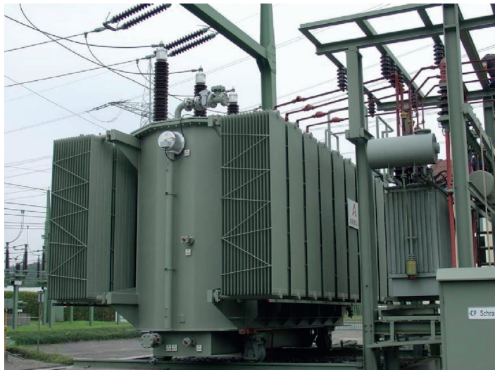
Figure 2: Hermetically sealed transformer
